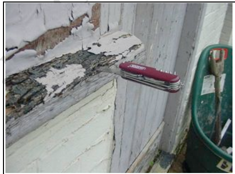
Lack of external painting
