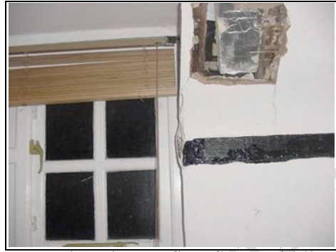
Deterioration to first floor middle room caused by work to roof
