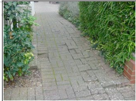
Areas of deterioration
