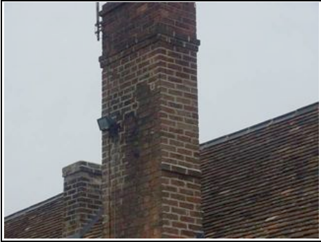
Weathering to chimney
