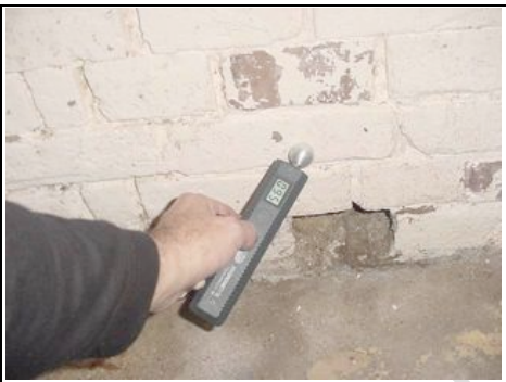
Very high damp meter readings generally and particularly to left side
