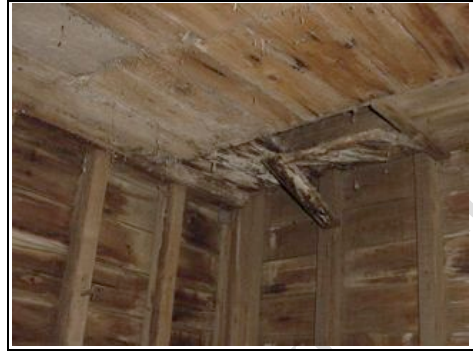
Wet rot, possibly dry rot to floor and walls
