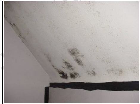
Cold bridging to left hand room
