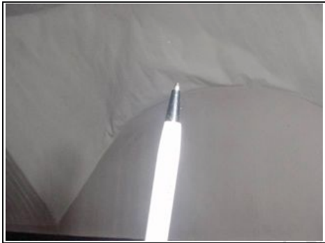
Dampness coming into eyebrow section of front right room
