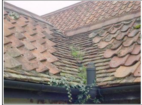
Vegetation growing from barn roof
