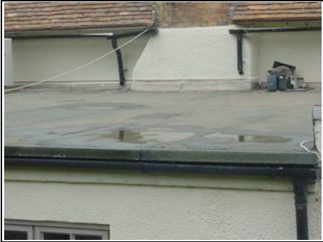
Ponding to flat roof
