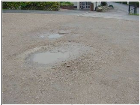
Deterioration to car park
