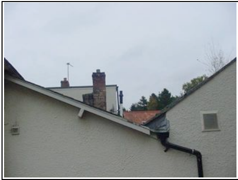
Defect to valley gutter to pub
